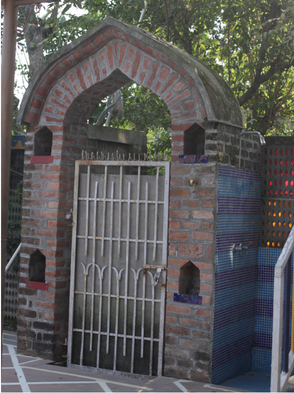
Fig. 22: Lacolas at different parts of the building of Chateau Garli, Garli, H.P.
